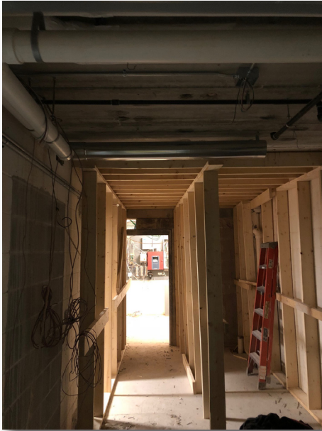
Shoring for the new floor in the original stair and elevator shaft.
