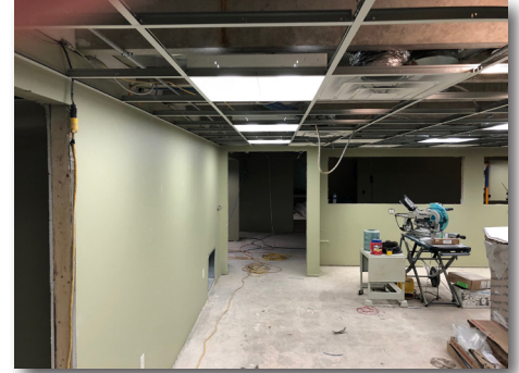
Ceiling grid and lights in lower level are starting to be installed.
