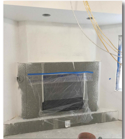
The hearth is prepared and ready to receive its mantel piece and stone veneer.
