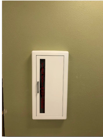
Fire protection extinguishers are located in the upper and lower levels. Fire protection sprinklers are ready for final testing.
