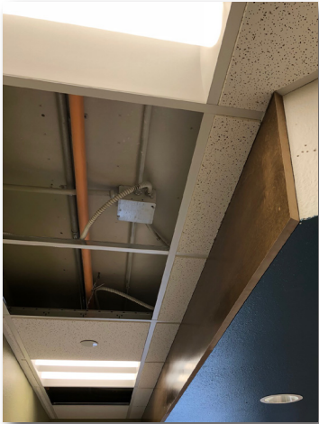
A look at the Circulation Desk soffit with its wood veneer cover piece. A bottom trim piece will be installed later to finish the look.
