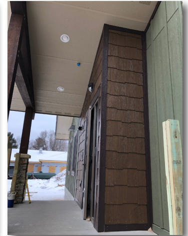
A look at the West entrance shakes. The West side of the building exterior siding is finished.
