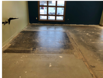
Construction crews are in the process of sealing the floor in the YA room in order to correct floor level on existing concrete slab.
